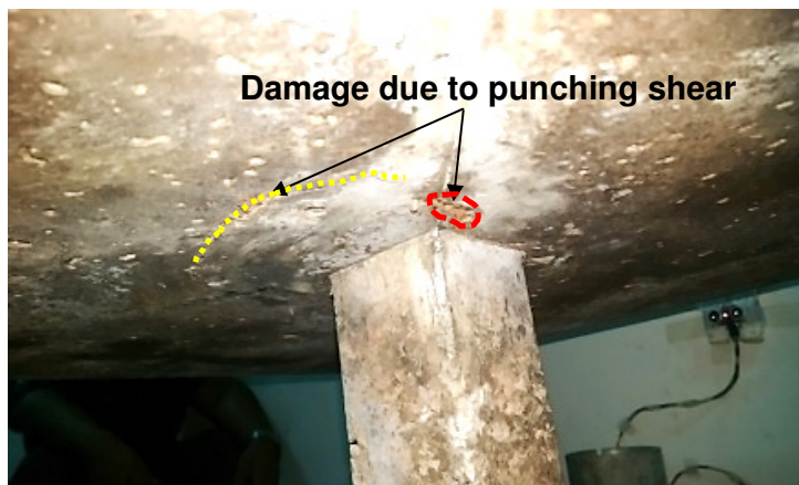
Figure10: Crack Formation of Flat Plate slab After the Dynamic Test
